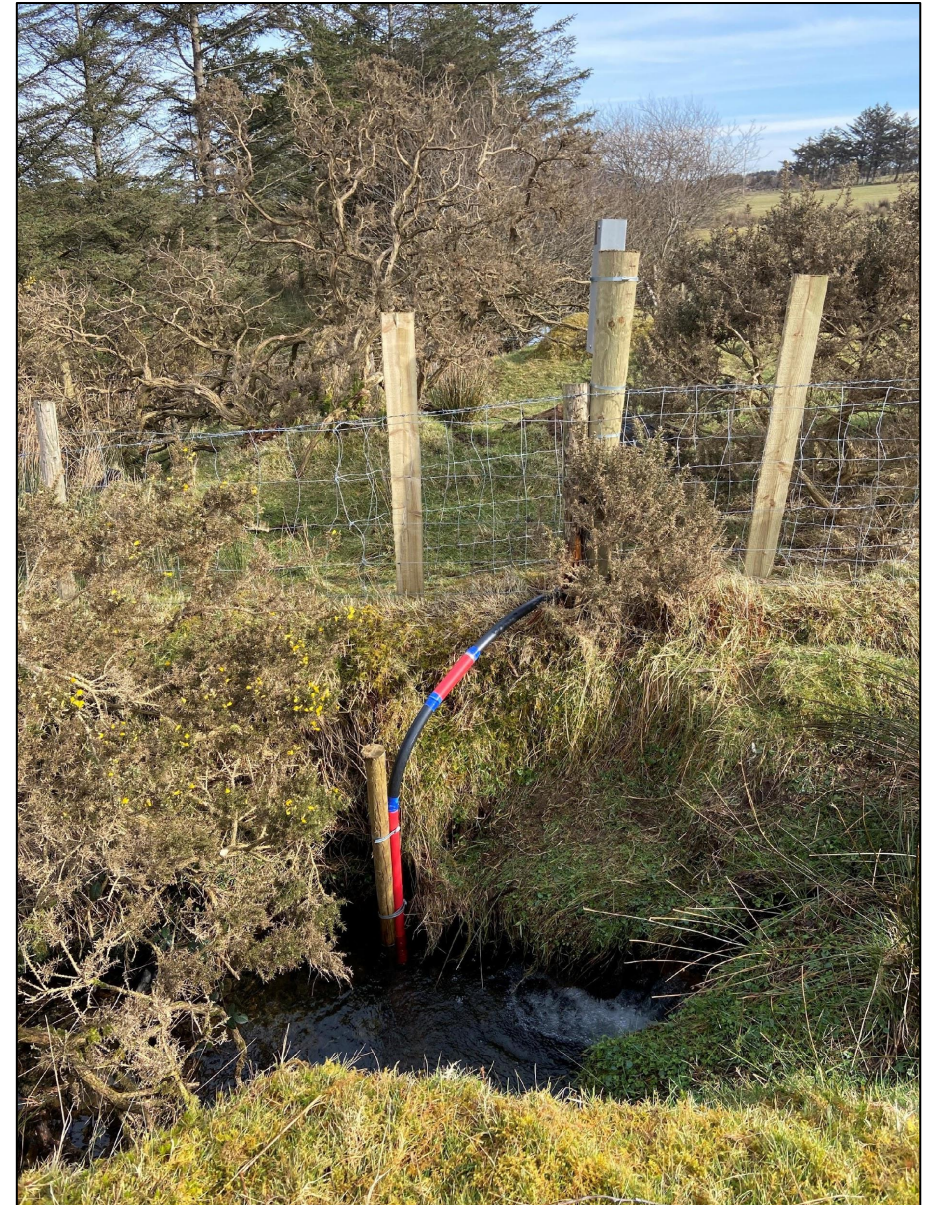
Monitoring equipment in place
